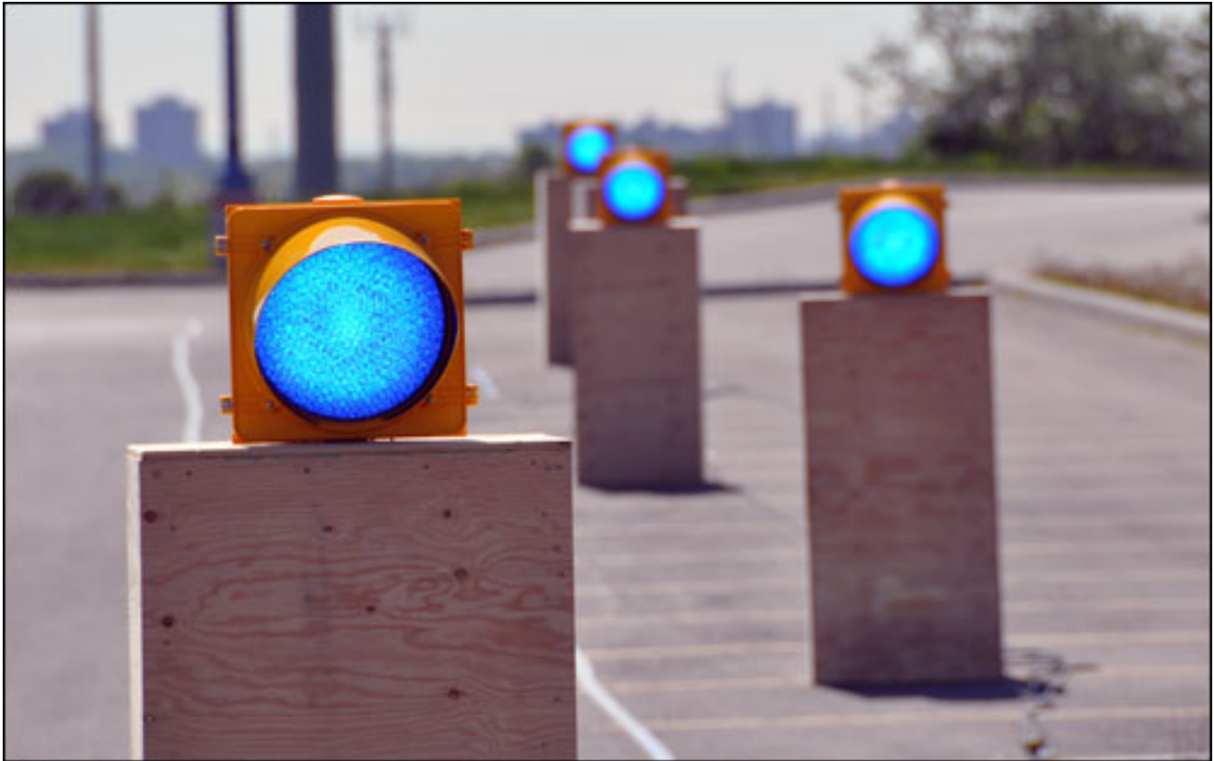
The lights used during the parking-lot trial were the same type of LEDs that the final system would employ to alert train operators to nearby track workers.
